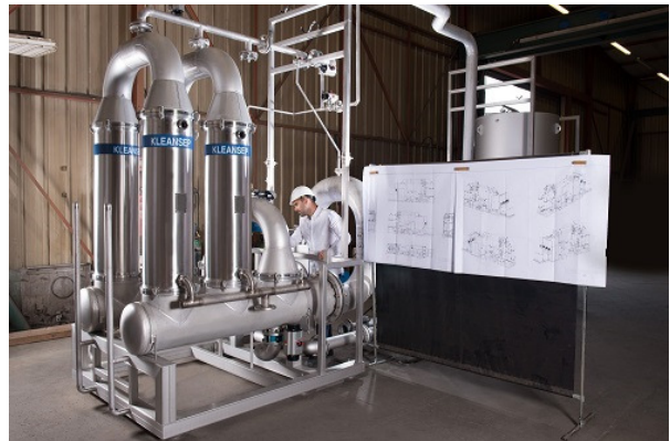
Industrial equipment and process engineering: filtration skid
